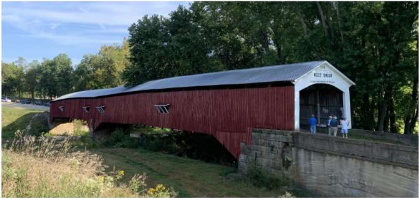
West Union Covered Bridge over Sugar Creek, Parke County, IN Built 1876 by Joseph J. Daniels Burr Arch truss, 315 feet, 2 span
